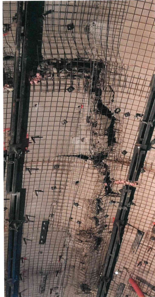
11 Overloaded segments in running tunnel 2 (TBM 1) Überbeanspruchte Tübbinge in Streckenröhre 2 (TVM 1)
